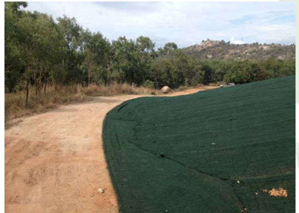
Synthetic erosion control matting to protect site until capping works begin in 2018
